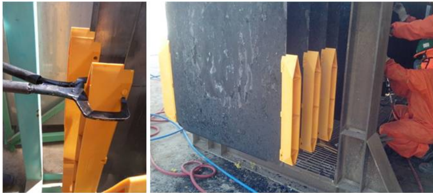
Figure 5: Installation of Idemin anode fittings at Lomas Bayas, Chile
